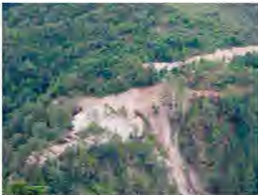
Figure 3.2. Landslide following road construction in Bhutan Courtesy: Patrick Durst.
