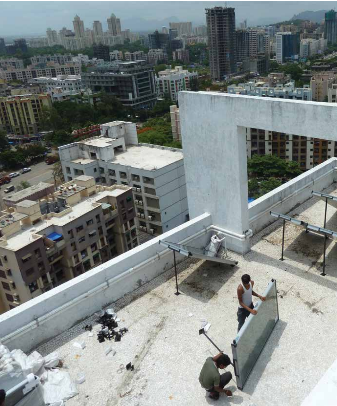
Installation of solar hot water systems in residential towers in Thane, Mumbai Metropolitan Region of India. In Thane it is mandatory by law for all new buildings to install solar hot water heating systems, which help reduce demand for fossil fuel-based sources of energy, mitigating adverse effects on public health and the global climate. Andrés Luque
