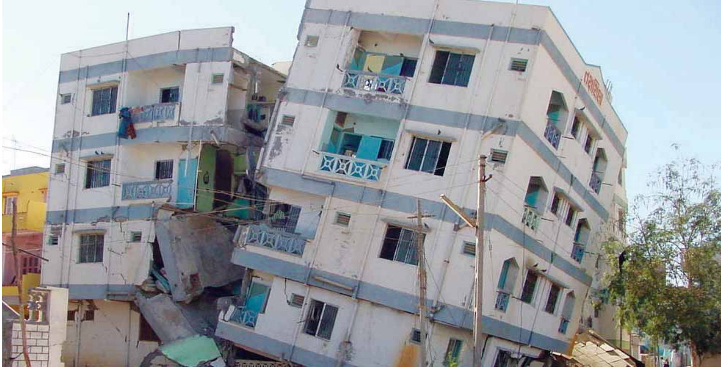
Damaged structure due to earthquake- Gujarat 2001
