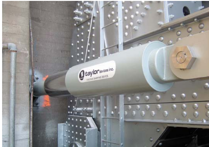
Seismic damper installed where the western portion (suspension spans) of the San Francisco-Oakland Bay Bridge meets Yerba Buena Island
