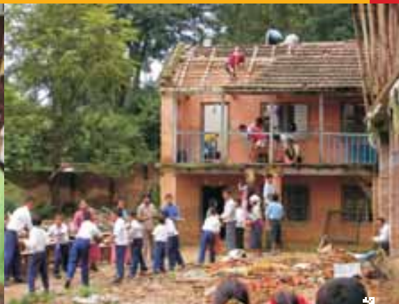
Community and school students involved in the demolition of the old school building (SESP)
