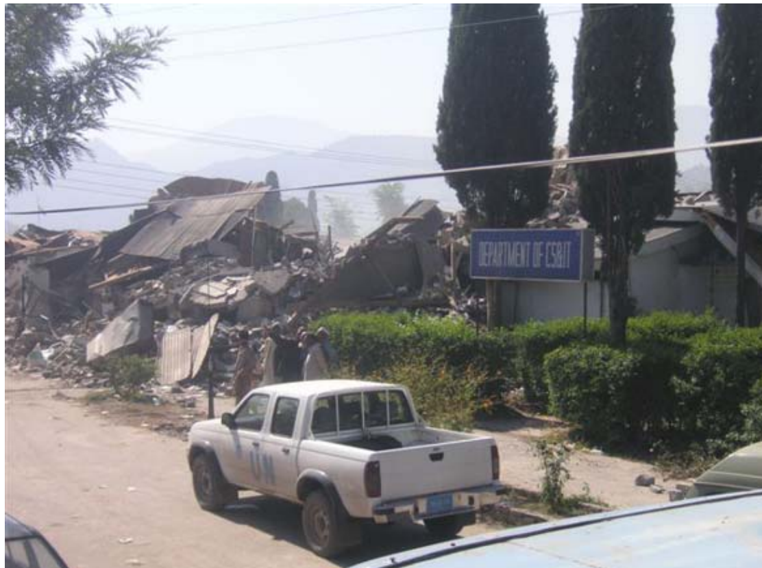
Collapsed public infrastructure (Photo credit : Roger Yates)
