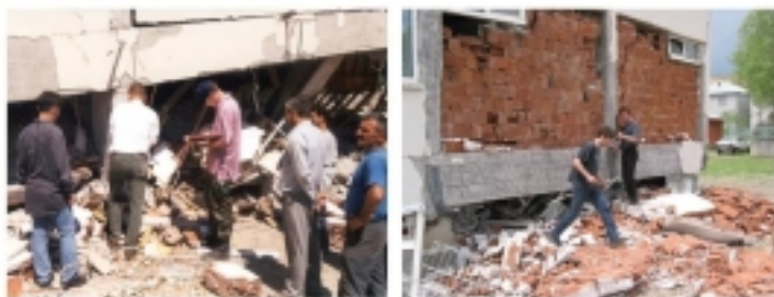
Figure 2. Documentation of structural damage by the engineering group of German TaskForce (EDAC staff) after the (left) 1999 Kocaeli and (right) 2003 Bingöl earthquake.
