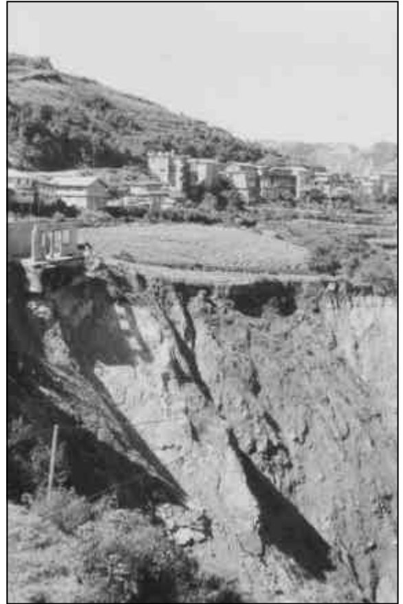
Erosion causes damage to buildings and agricultural land
