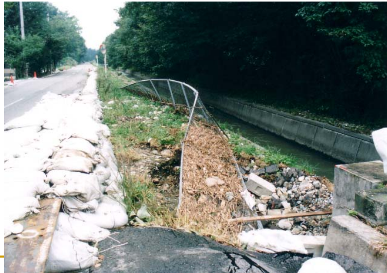
No.3 Damage of the irrigation canals
