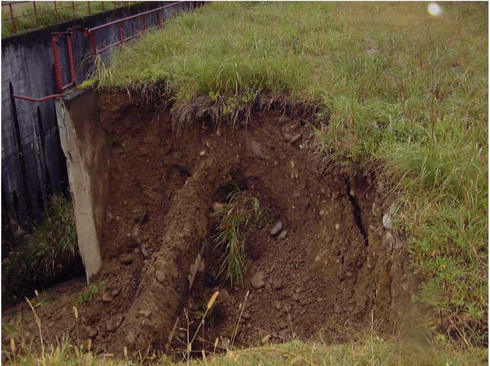
Cave-in in spillway
