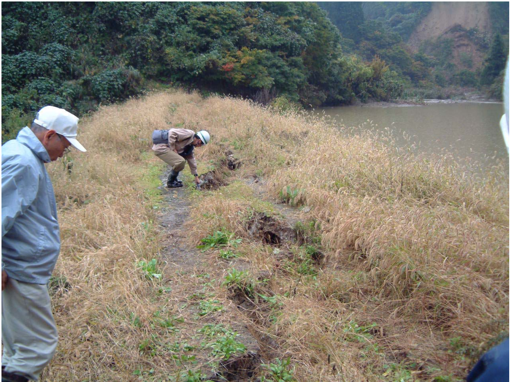
Crack on embankment of irrigation pond
