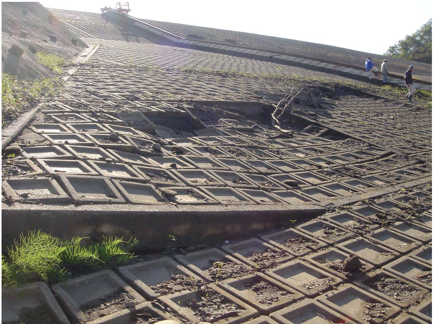
Damaged Dam and Irrigation Pond (Kawanishi Dam)
