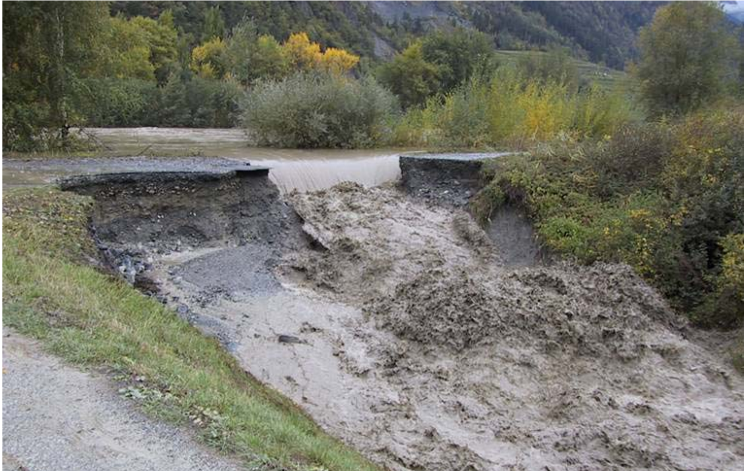
Old and fragile flood embankments
