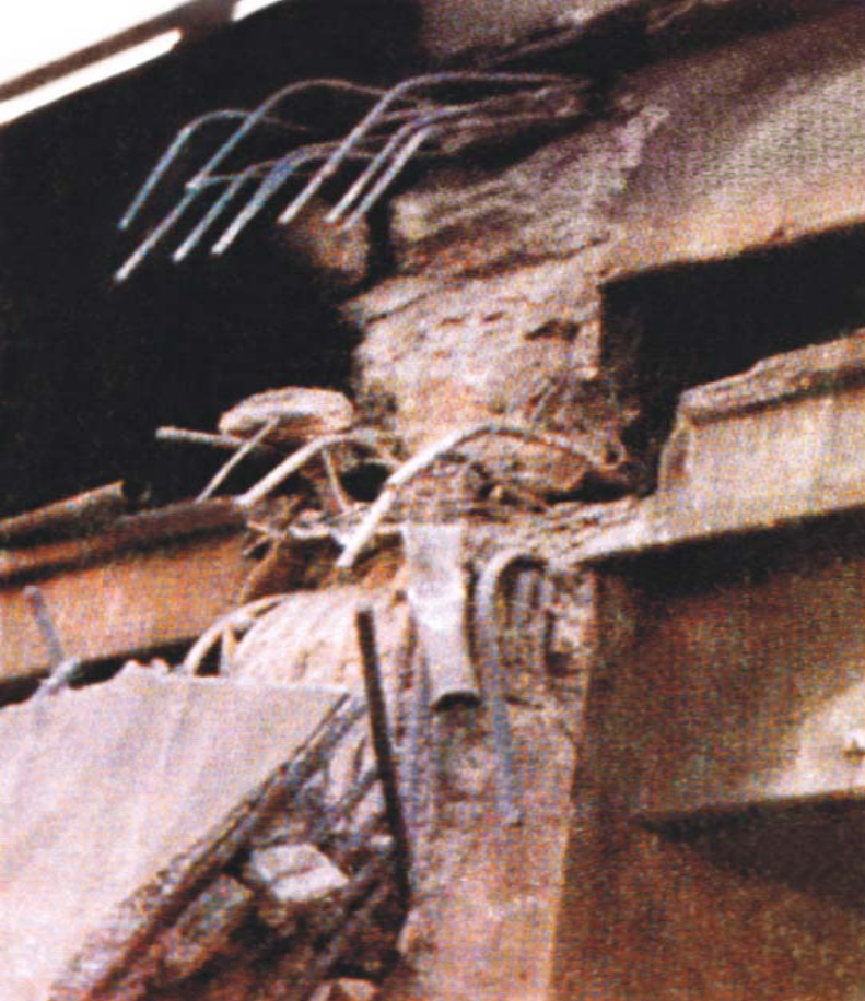
Failure of an elevated highway in San Francisco, CA. Loma Prieta EQ 1985
